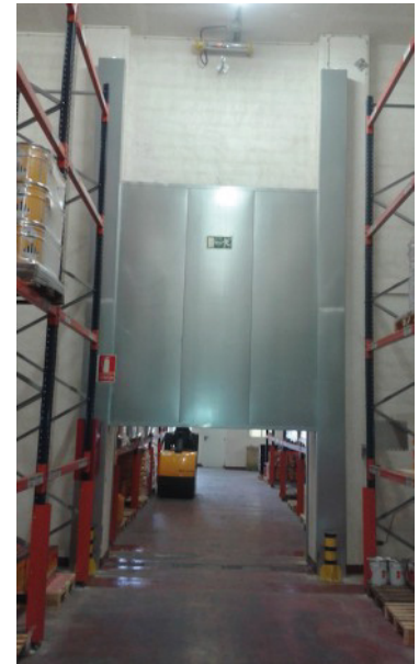
▲ Vertical climbing guillotine door with electromagnet closing system and counterweight
